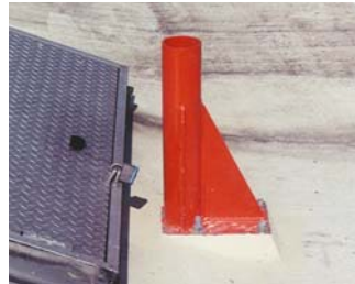
Permanent Davit Base—Figure 2
